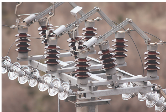
Can you see the dark red-brown ceramic electrical insulators?
