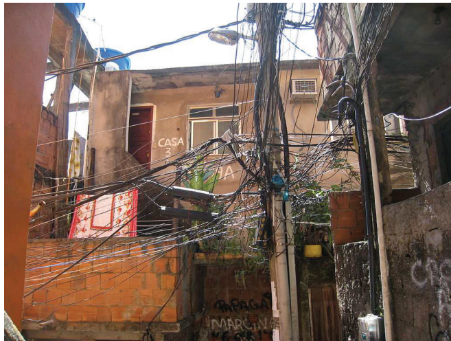
Look at this mess of illegal electrical connections. 4
