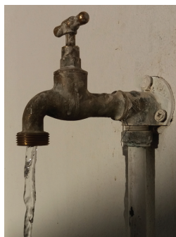
Clean water coming out of the tap. 1
