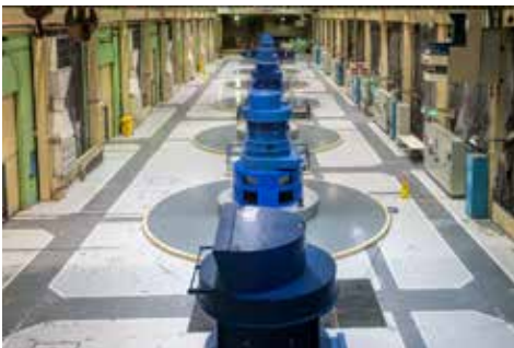
Figure 18.9: The generators inside the hydroelectric power plant.
