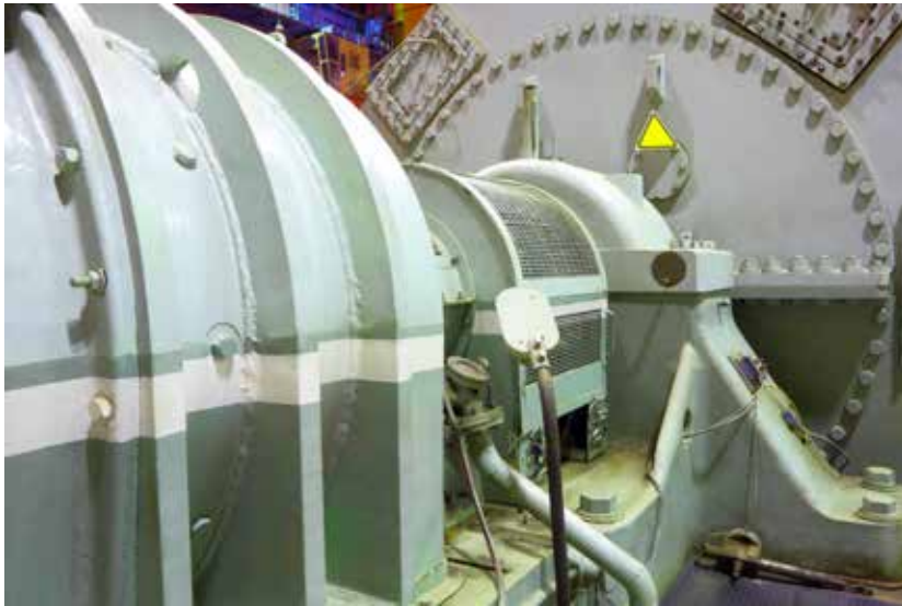
Figure 18.4: A modern-day steam turbine connected to a generator.
