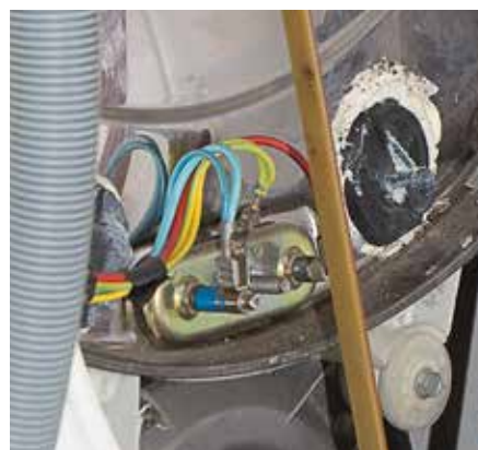
Figure 17.3: The green-and-yellow earth wire connected to the metal casing inside an electric motor.
