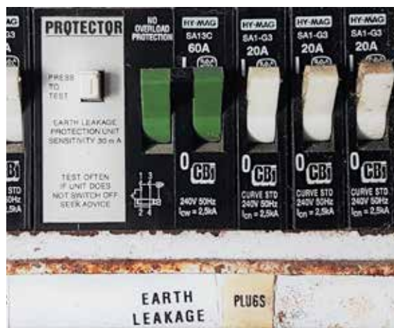
Figure 17.9: An example of the earth leakage and main switch on a distribution board in a house.
