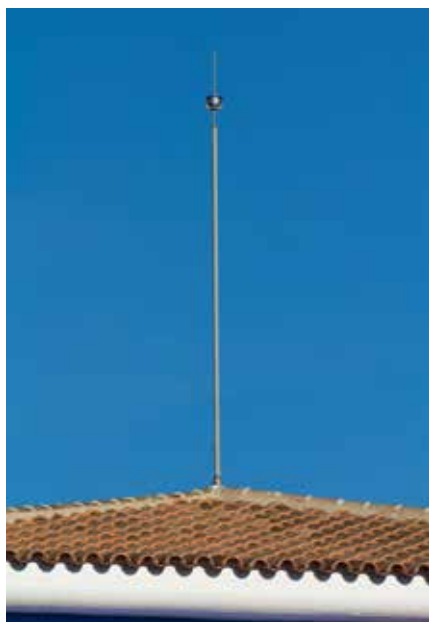
Figure 17.10: A lightning rod on the roof of a house.
