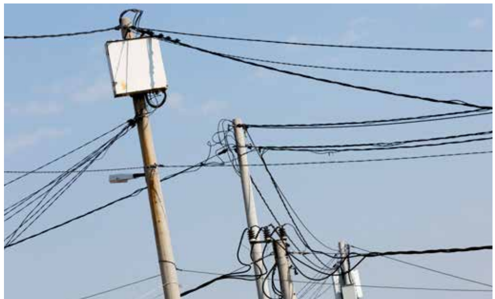
Figure 17.14: Electricity theft is illegal and also very dangerous because of the insecure connections
